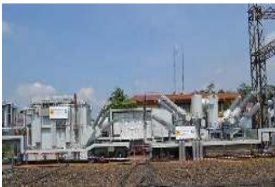
Gbr.1 Mobile Substation 150/20 kV
