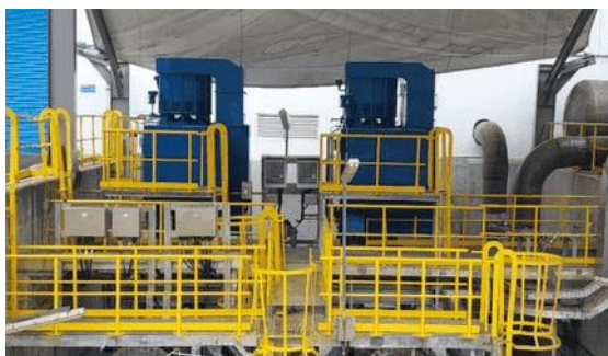
Gambar 5. Hotwell Pump Unit 3 Ulubelu [8]
