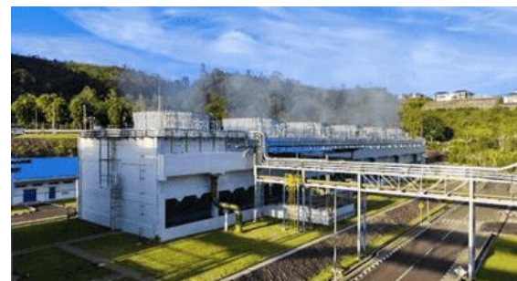
Gambar 4. Cooling Tower Unit 3 Ulubelu [8]
